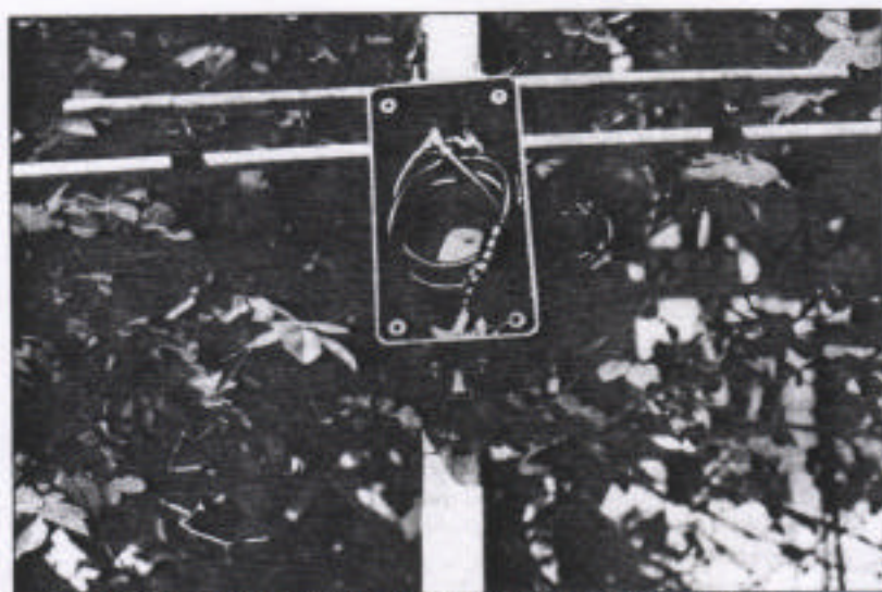
Photo B. Close-up of balun box. Note the "T" match bars and the driven element.
